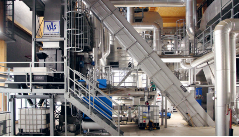
ABB: ecological heating systems thanks to district heating with local wood.
